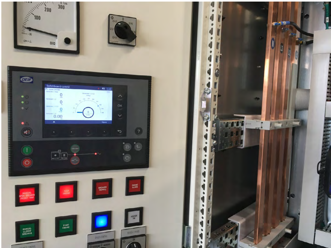
Power Management unit in the switchboard
