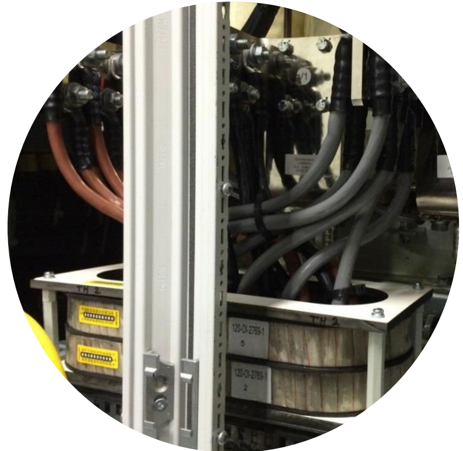
Fig. 5: two assembled cores in the cabinet
